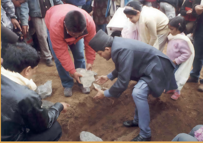
The foundation stone was laid in 2003. The Minister of Health, Dr. Upendra Devkota, laid the first stone of the hospital.
